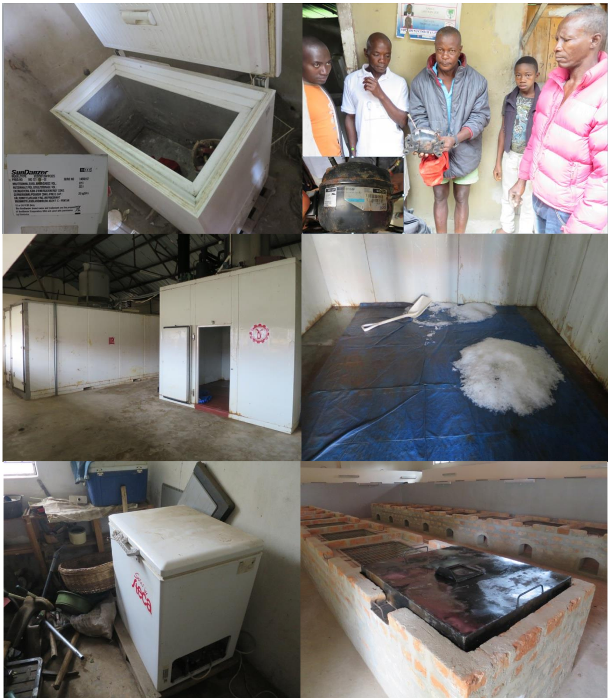
Plates 4.15a-f: Clockwise from top left a&b: Failed Sundanzer ‘solar’ (12-24v DC) refrigerator York, Island due to ‘faulty compressor’, c&f: Non-operational cold-rooms Bonthe fisheries centre, e. Faulty solar freezer belonging to project member, awaiting shipment of spare-parts d. Fuel efficient fish smoking systems Bonthe fisheries centre with no community uptake as yet
